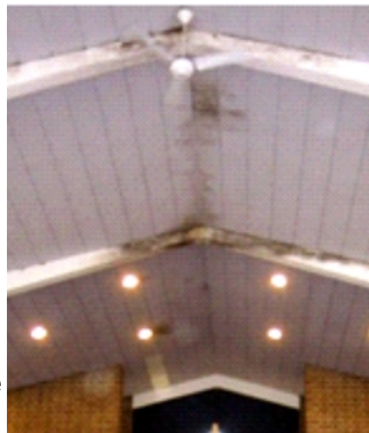
Unfortunately the damage to the roof can be seen clearly inside the building.
